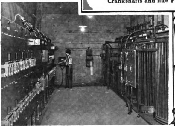
B—The Entire Plant is Operated by Electric Motors. This is a View of the Main Switchboard and the Battery of Transformers from which the Electric Current is Taken
